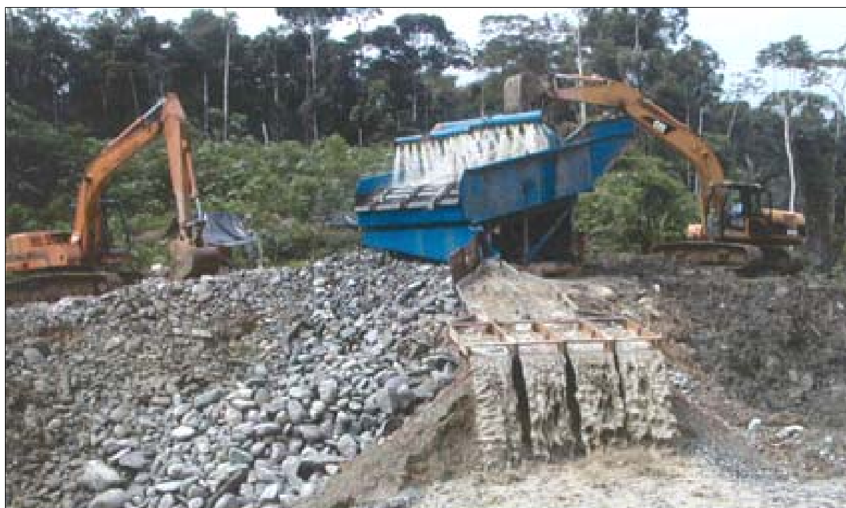
Derocker Gold processing plant, sluice and loader in operation at HCR's PF #1 mine in Ecuador
