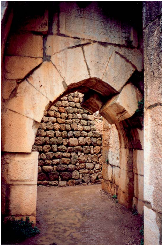
Figure 8 This is an example of a slipped voussoir in the Crusader fortification of Kala'at Namrud. Note how base of one side of the arch slipped outward, allowing the voussoir to drop.
