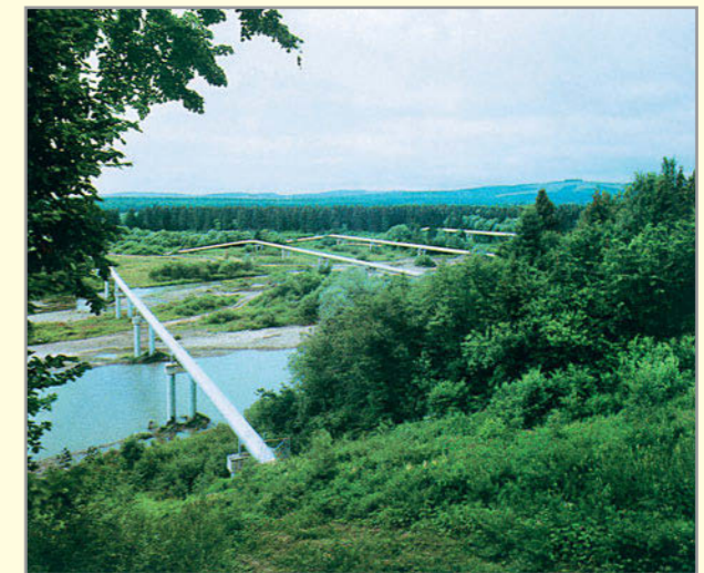
An array of natural gas pipelines crossing a river
