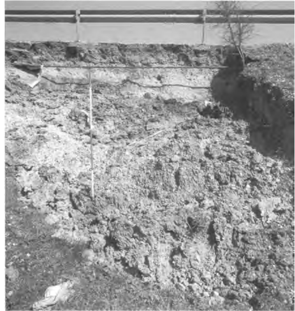
FIG. 10.5. Failure of a clay fill.
