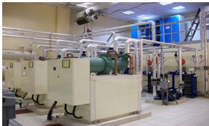
Figure 4. The heat pump modules (general view).
