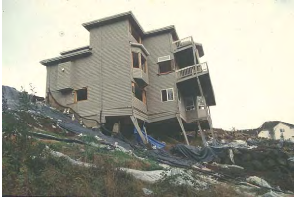
Figure 4 Slump destroys a house in Tigard, Oregon, USA; note deformation of supporting pillars. This home was built on the toe of an ancient landslide that reactivated in February 1996.
