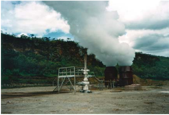
Fig. 104 A geothermal energy producing field at Olkaria near Lake Naivasha.
