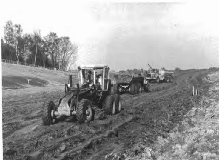
Fig. 1. Temporary excavations in the Wittering & Earnley Formations, M27 motorway, Dummer's Copse, West End, near Southampton, Hampshire, 1983.
