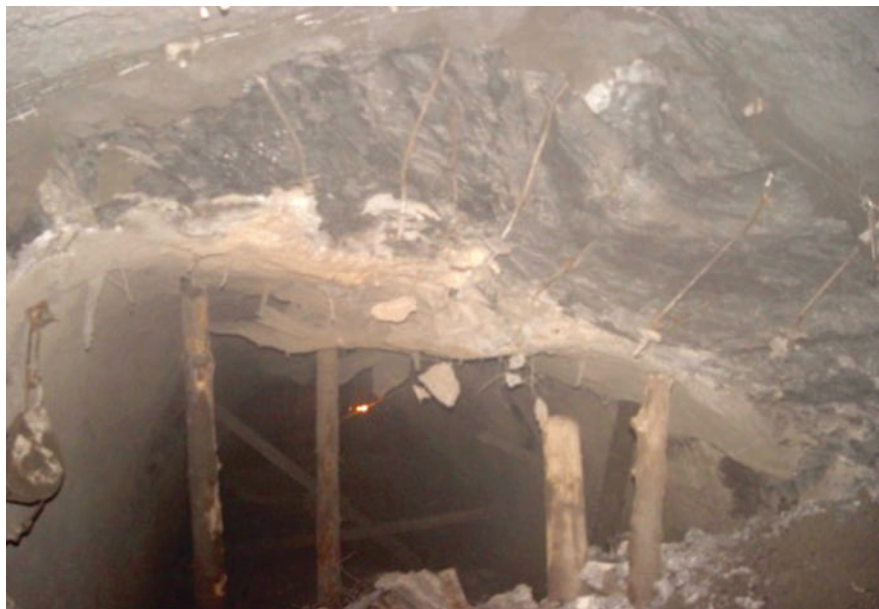
Fig. 7.9 Roof subsidence of the heavy vehicle line roadway (He et al. 2012)
