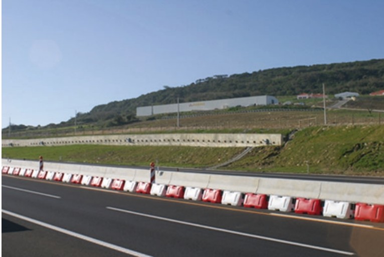
Fig. 4.27 General view of the section at the end of the slope stabilization works
