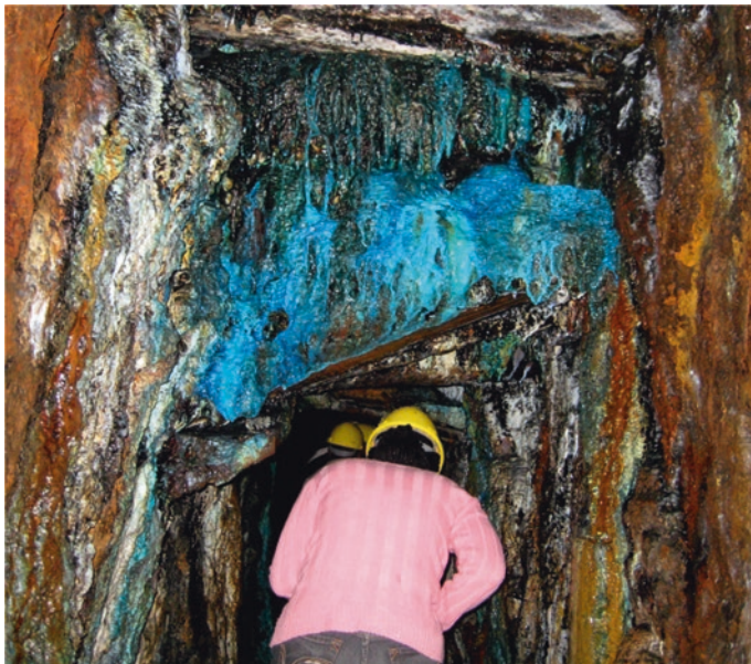
Fig. 11.3 Acid groundwater causing deterioration of rock mass and steel support in a mine tunnel. Oxidation of metal sulfides by oxygen-rich percolating groundwater caused forming of sulfates and acid water. The blue and white stained areas are sulfates precipitated from seepage water (Gold, silver, copper, and lead mine Rammelsberg, Goslar, Harz, Germany; photo courtesy S. Carelsen 2010)
