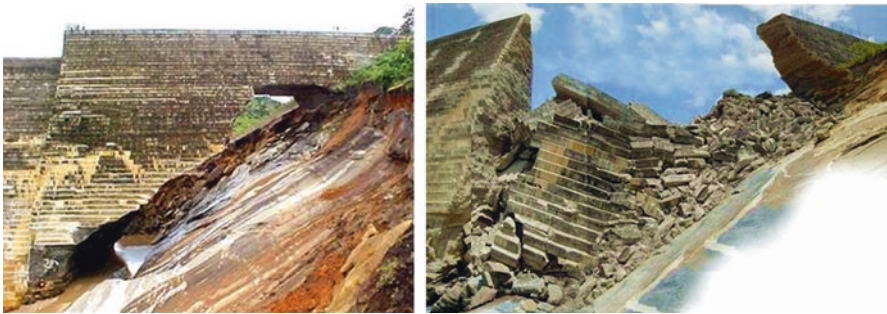
Fig. 24.14 Left abutment of Camará Dam. Just after failure on the left side, and few days later, a complete concrete collapse
