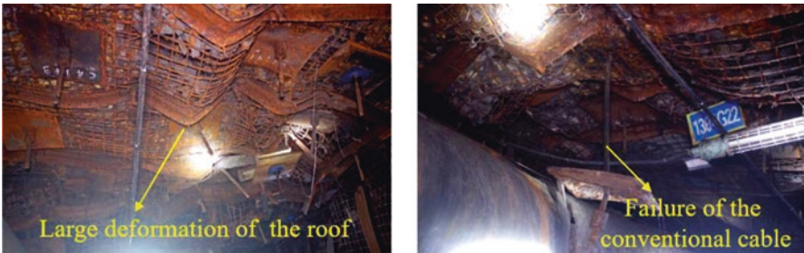
Fig. 17.23 Large deformation of the roadway surroundings in a deep coal mine
