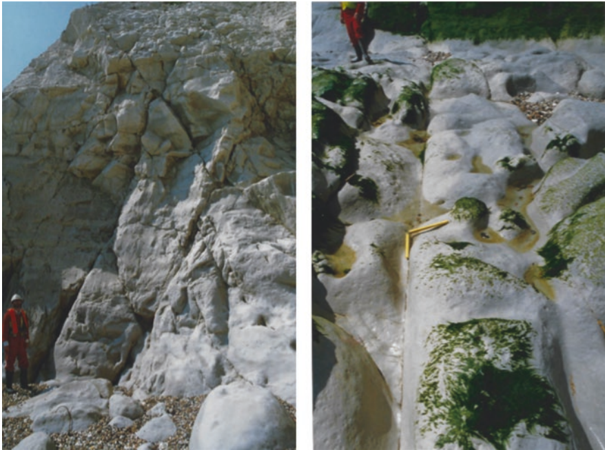
Fig. 18.1 Left: Representative conjugate jointing and sub-horizontal bedding in the grey chalk at Shakespeare Cliffs. Right: Joints in the underlying chalk marl where the tunnels were to be constructed. Note the extreme planarity of the joints, which was responsible for extensive overbreak in permeable, lower-cover sections
