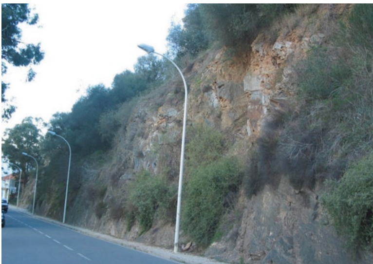
Fig. 4.29 General view of cut slope located at EN120 motorway in Odemira, Portugal
