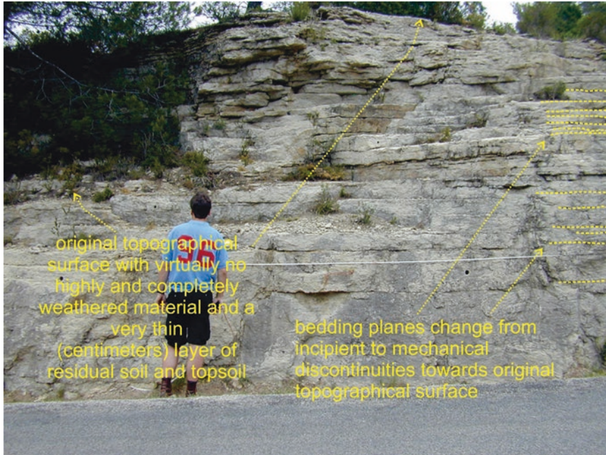
Fig. 11.4 Decrease of spacing between mechanical discontinuities ( banking spacing) nearer to the original topographical surface due to weathering of incipient bedding plane discontinuities into mechanical discontinuities. Note the very thin layer of weathered material and topsoil derived by weathering from the limestone rock mass that consists of fairly pure calcareous material (cut slope along road T322-Montroig to Colldejou, 1.3 km SE of Colldejou, Falset, Spain; photo courtesy W. Verwaal 2001)
