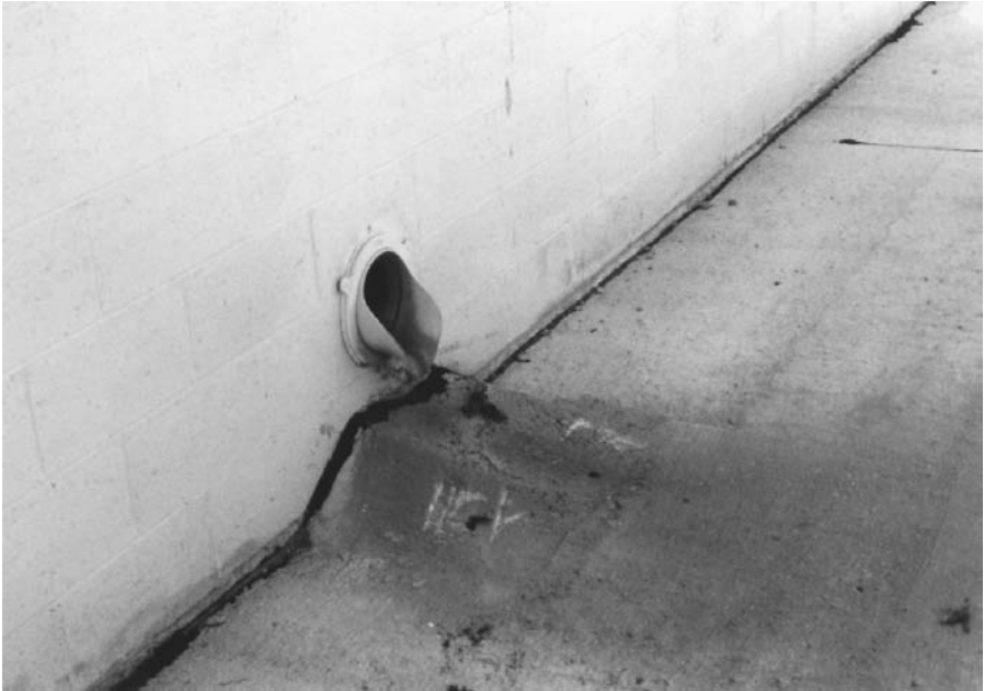
FIGURE 13.6 Improperly placed drain outlet.
