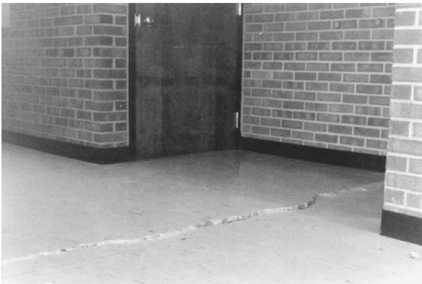
FIGURE 15.4 Floor crack due to creep of twin-tee concrete slab.
