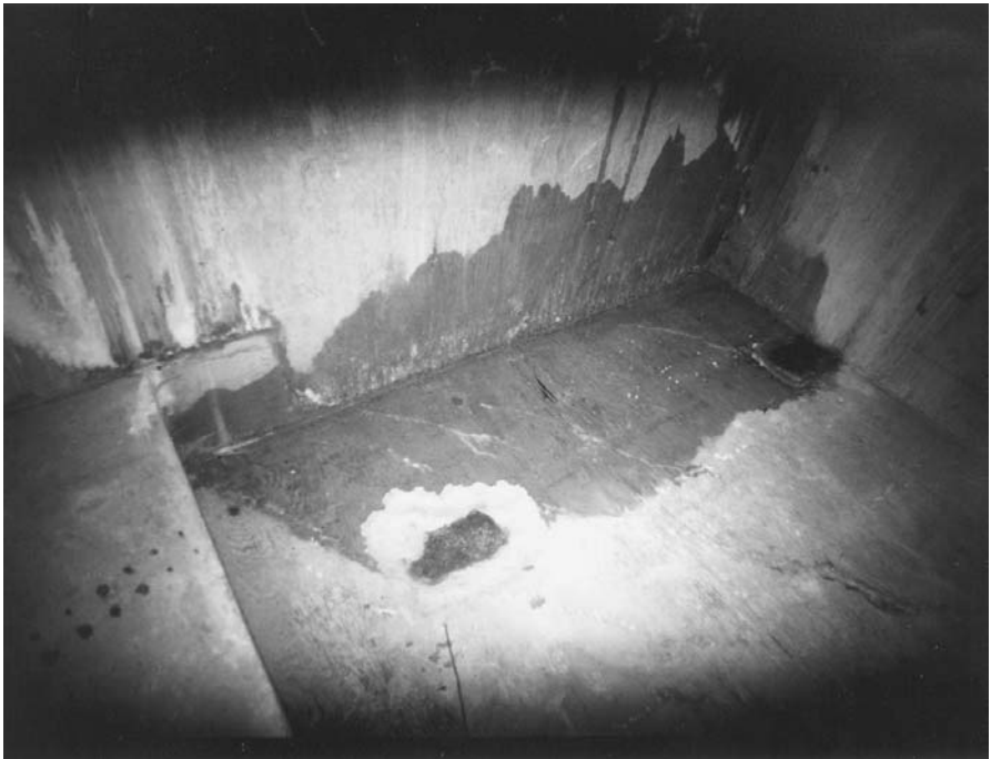
FIGURE 15.1 Water seeped into the lower floor.
