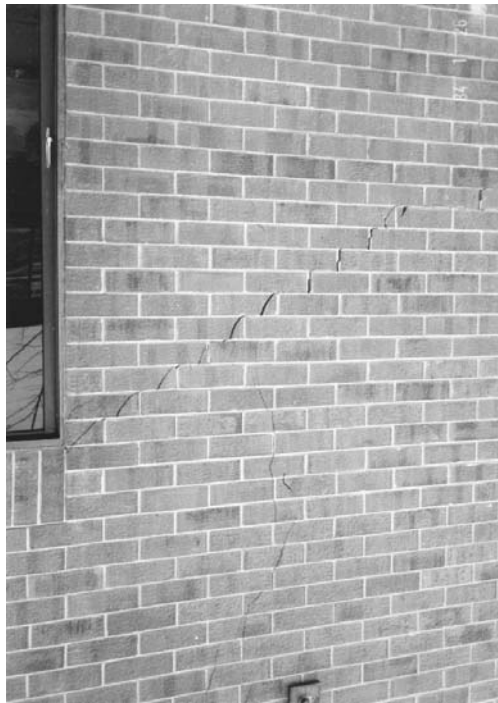
FIGURE 15.3 Cracks due to temperature in massive brick construction.
