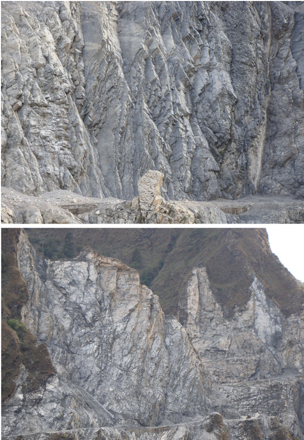
Fig. 12 Railway bridge-site access road in Indian Kashmir. An illustration of slope limits pushed by ‘favorable-in-the-circumstances’ (hard rock) bedding-plane and joint-dip angles. Safety of access during heavy rain is frankly doubted. Slope formed by downward excavation from valley-side footpath 20 to 70 m above this final access road. Note scale of tractor in right-side of lower photograph
